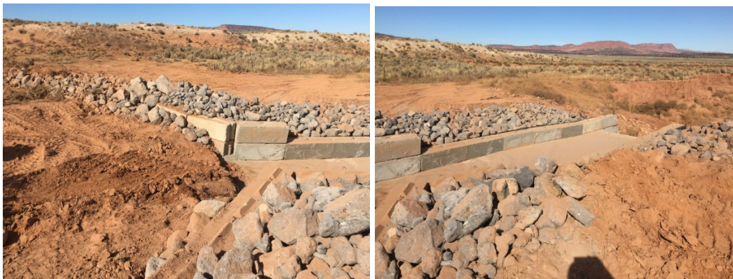
Figure 13: Upper portion of headcut where water will flow into the now stabilized headcut.
